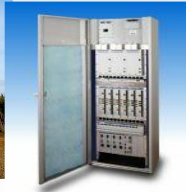
Macrocell BTS radio cabinet hosts TX/RX
