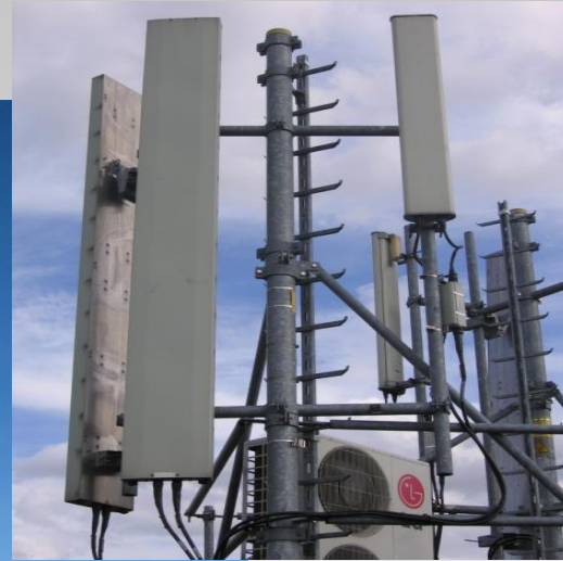
BTS antenna system
