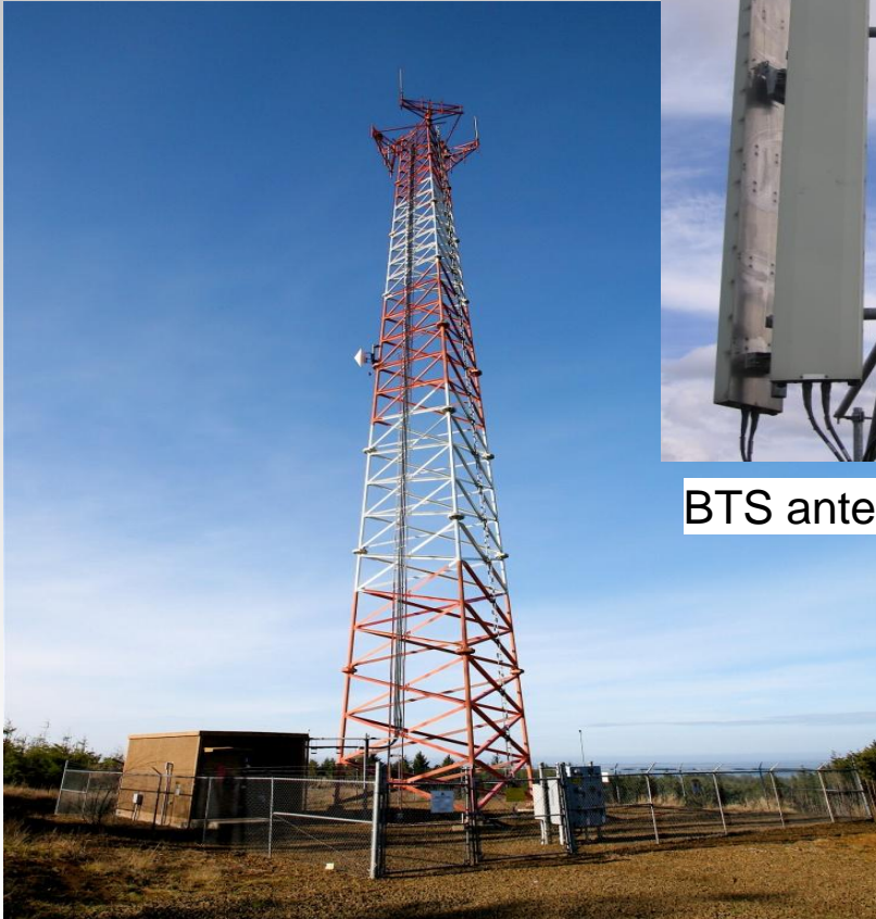
Typical BTS installation
