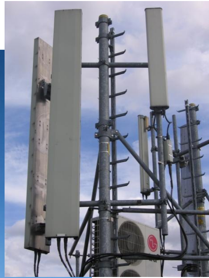
BTS antenna system
