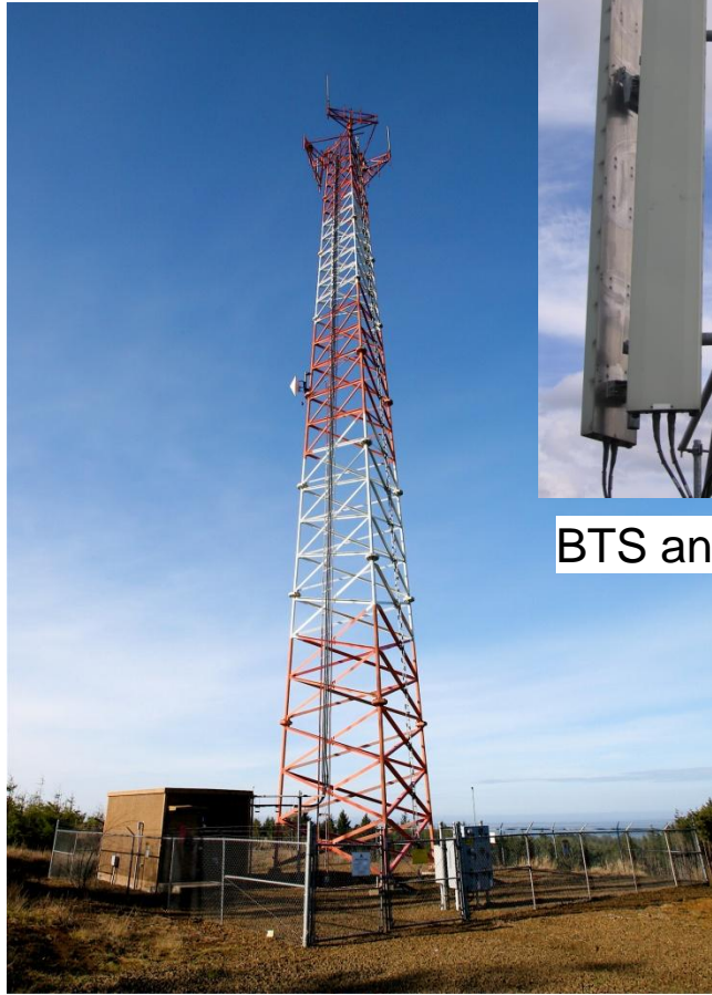
Typical BTS installation
