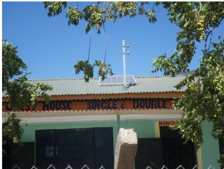
Figure 2.3: Grid disconnected and PV panel installed instead. Picture taken by Prof. Josef Noll in the village of Selela, Tanzania
