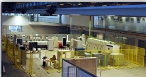
Figure 5-6: TECNALIA Laboratories (INGRID)
