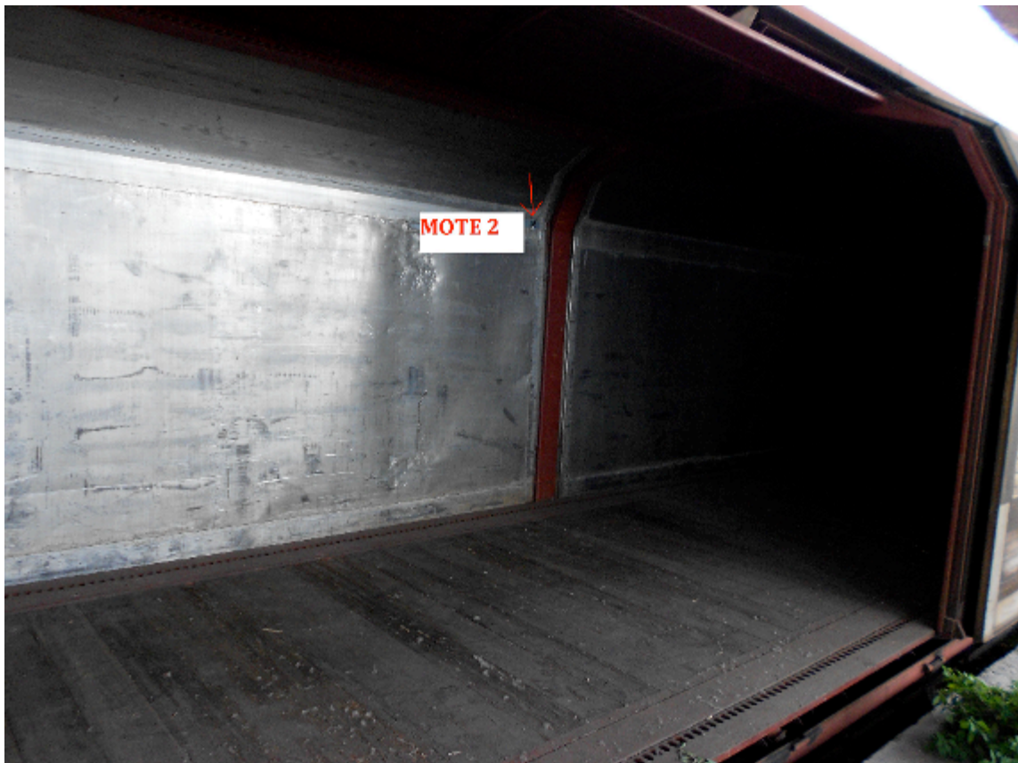
Figure 32 Inside of car mote 2
