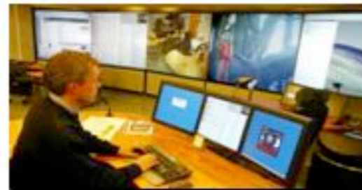
Control room offshore
