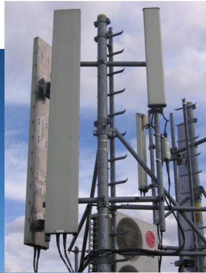
BTS antenna system
