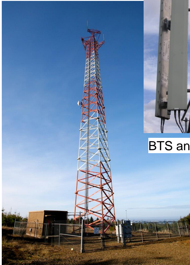
Typical BTS installation
